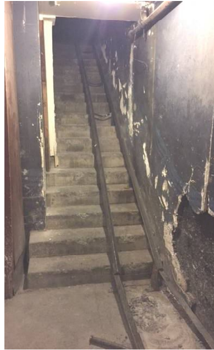
The rails on the stairs are used today to roll the beer kegs down.
